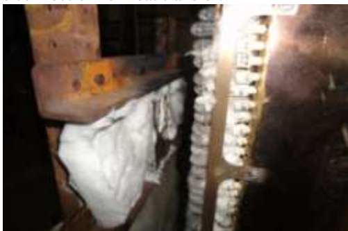
Fig. 22 Infra-red lamps, close-up view
